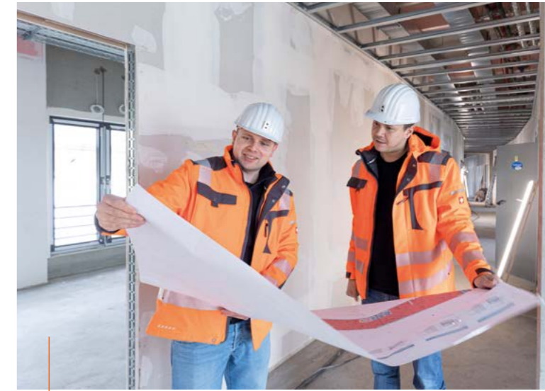
Morsleben repository: Shell of the new administrative building. Konstantin Bochmann and Marcus Eggstein examine the next lot of plans for its interior finishing.
